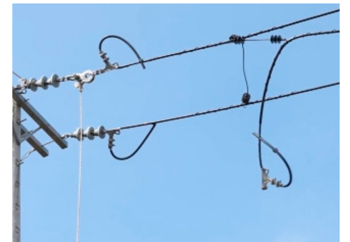
The device holds the power line in place, preventing it from falling to the ground.
