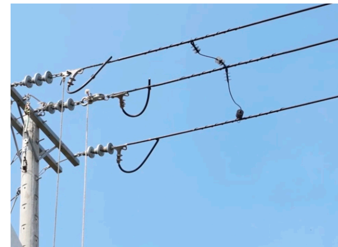
The two components of the cable support safety device are attached to the power lines.
